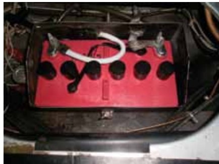
Electrical system and cables.
